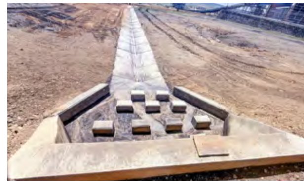
Water management, Shondoni Coal Mine, Embalenhle | Sasol Mining
